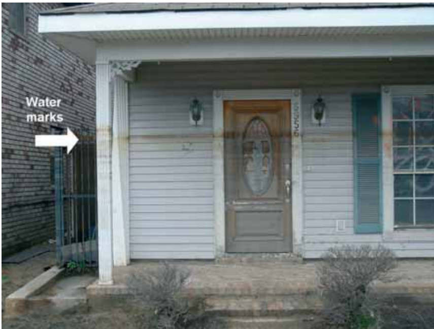
Figure 8-4: Water marks on a building near the breach in the 17 th Street Canal.
