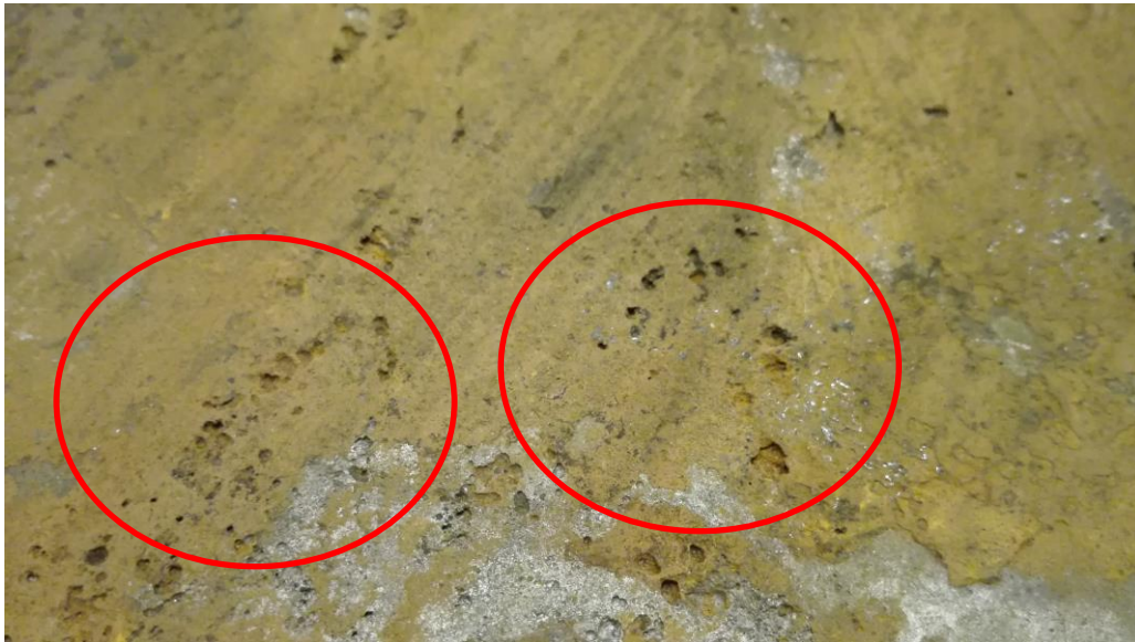
Figuur 5-1: putcorrosie dieseltank Oldebroek
